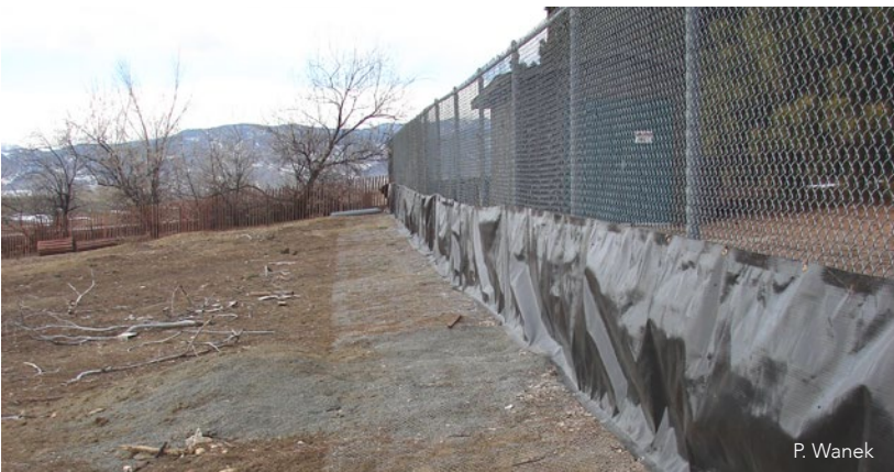
Modified existing chain-link fence to inhibit movement back into park. (prairie dog side)
