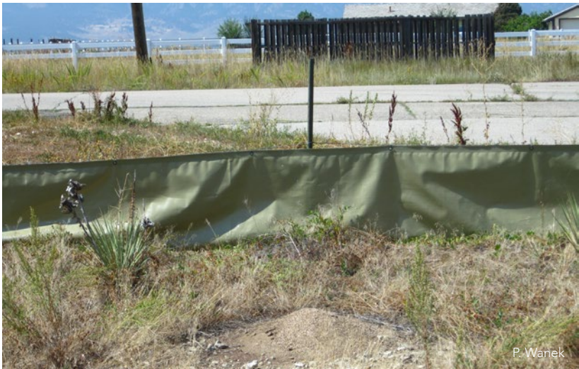
Flawed vinyl barrier installation.
