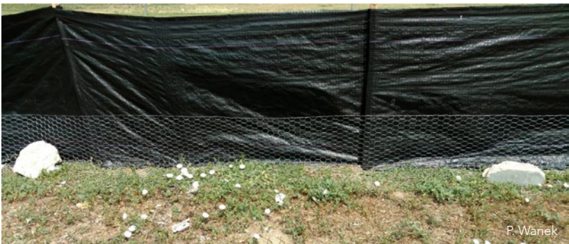
Modification: Using two-foot wide one-inch netting poultry wire, lip one foot vertically and use a staple gun to attach to wood posts. Anchor horizontal piece to ground with six-inch pins.
