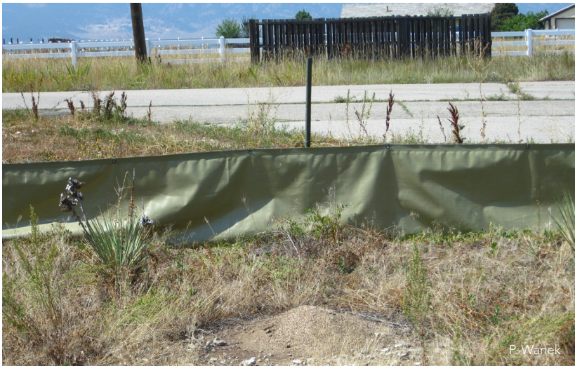
Flawed vinyl barrier installation.
