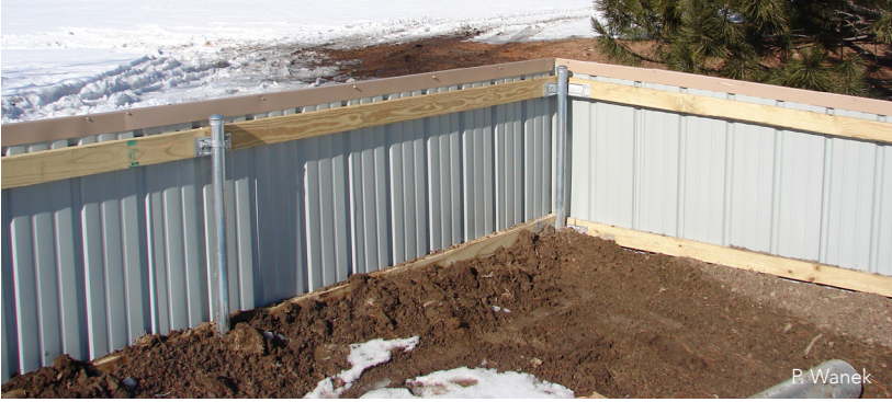
Prairie dog side of barrier. Note wildlife safe caps on metal posts and elongated cap along top of metal fencing.
