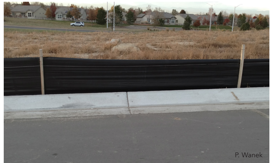
Silt fence with stakes and staples exposed.
