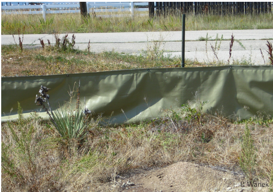
Flawed vinyl barrier installation.
